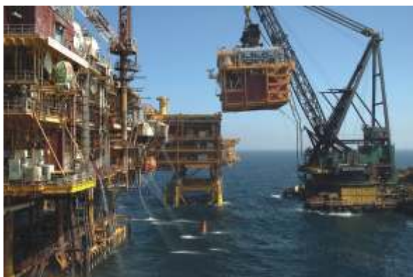
An offshore production facility in Mumbai High
